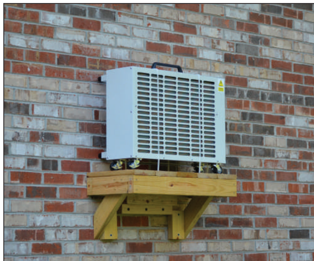
Outdoor Heat Exchanger*
