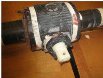
Figure 4-10 Close-up of Valve Operator and Remnants of Actuator Nut
